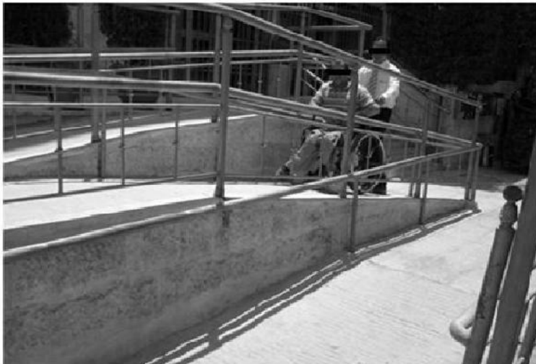
Figure 5. Photo of a substandard ramp in the entrance of HCD main office.
