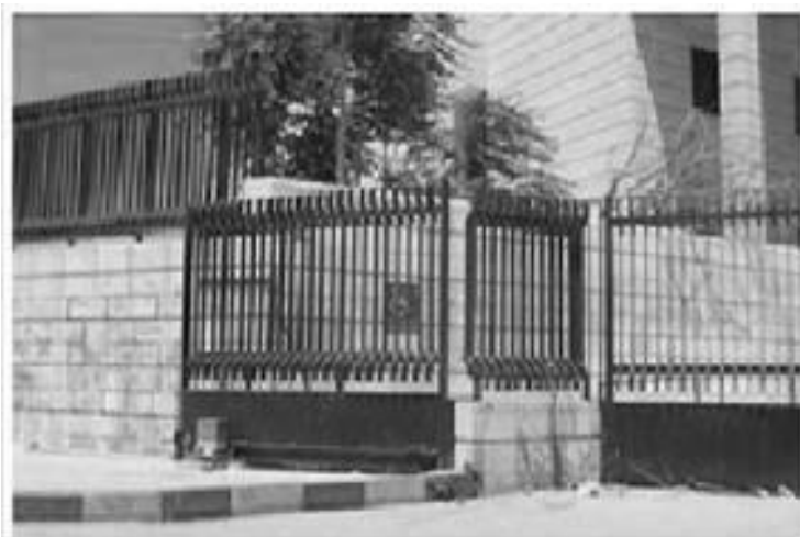
Figure 4: Photo of no ramp to connect the main road to the gate of the stadium.
