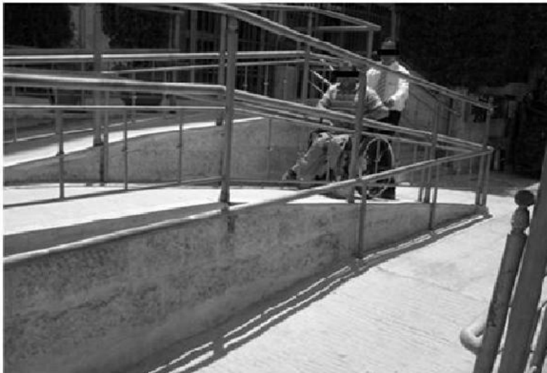
Figure 5. Photo of a substandard ramp in the entrance of HCD main office.
